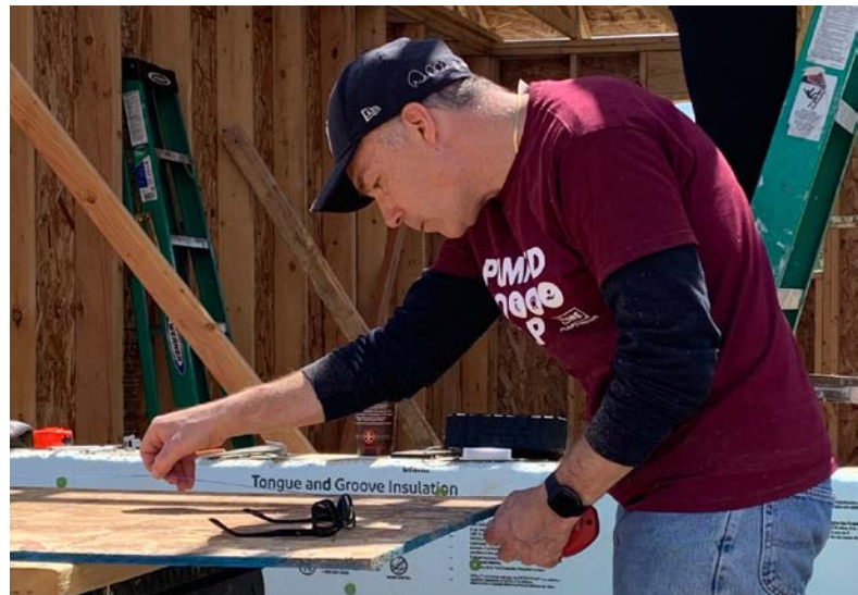
Crane Pumps & Systems associates in Piqua, OH working with Habitat for Humanity to build an affordable home in their community.
